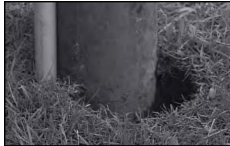
Faulty annular seal.
