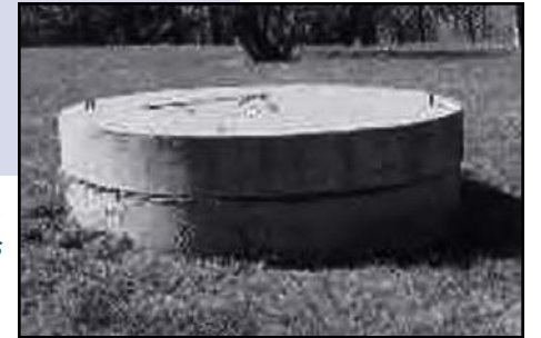
Well pit with concrete cover. Credit: BMP: Water Wells
