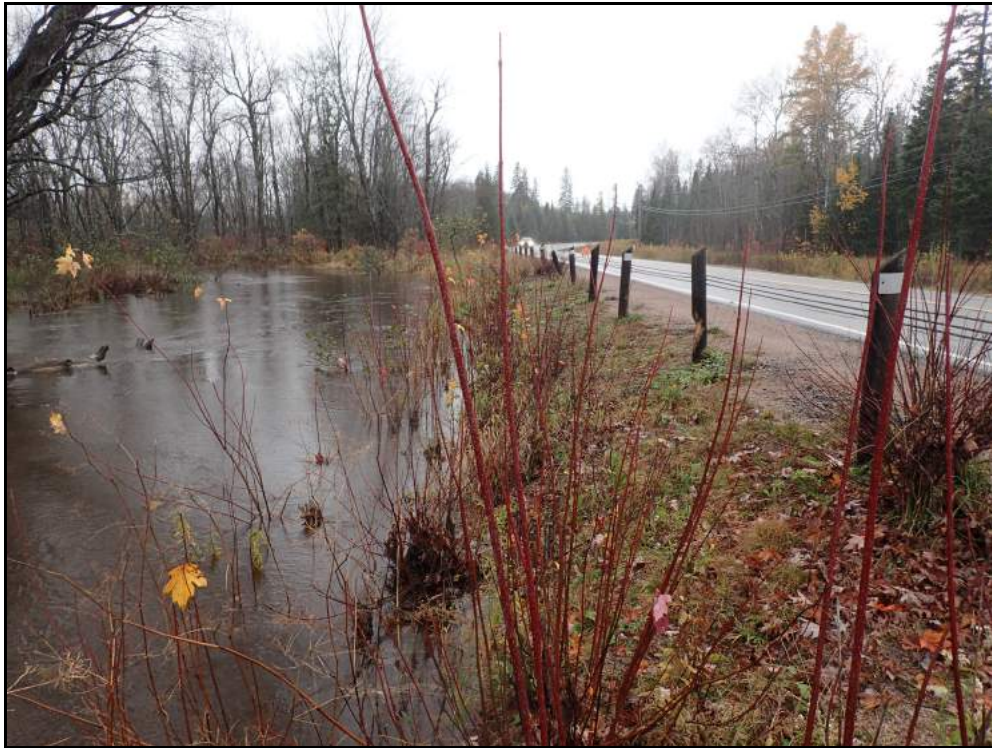
Figure 3.8: Wasi River Reach C-3 – Beaver damage to guardrail posts.
