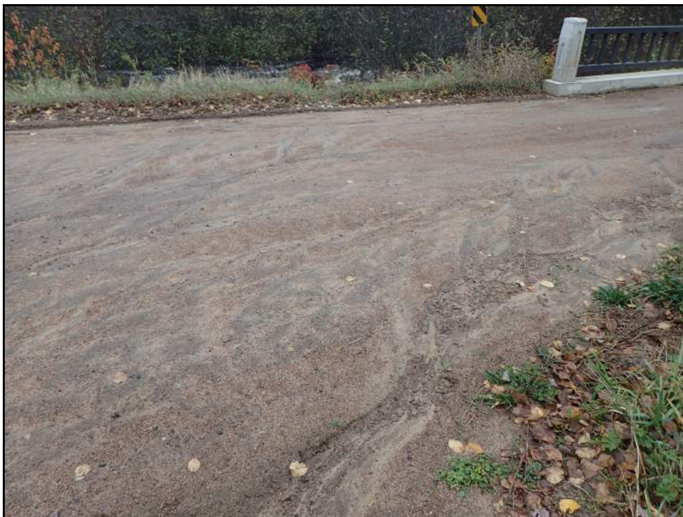
Figure 3.11: Sand erosion and transport towards Wasi River at Wasing Road.
