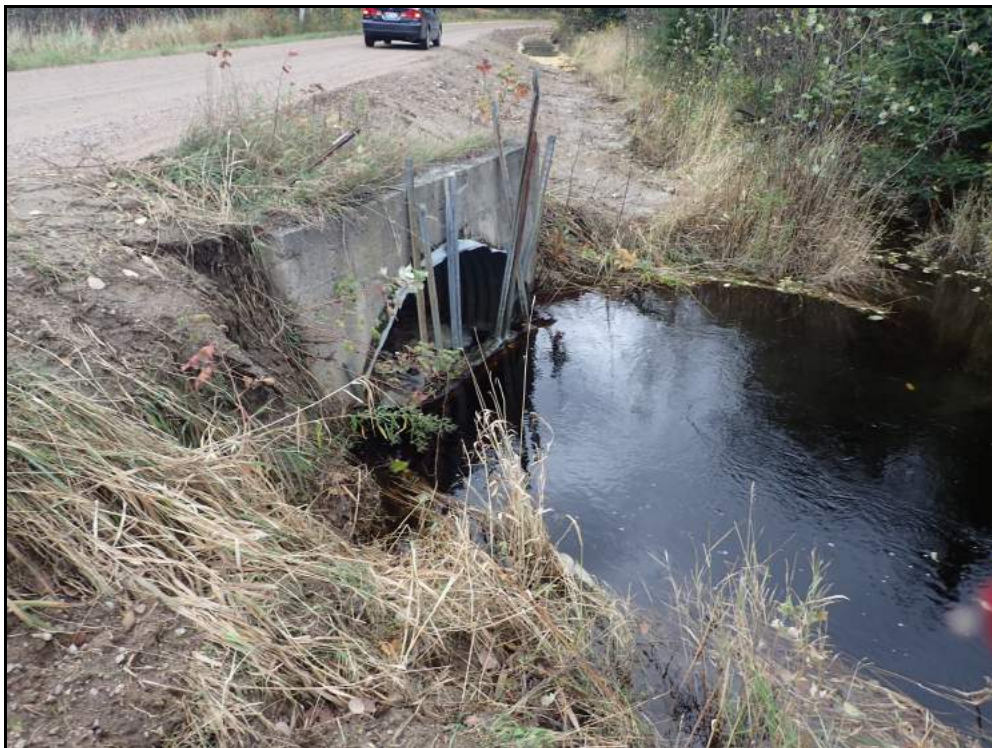
Figure 3.13: Sediment discharge from roadside ditch to Graham Creek – Maple Road.
