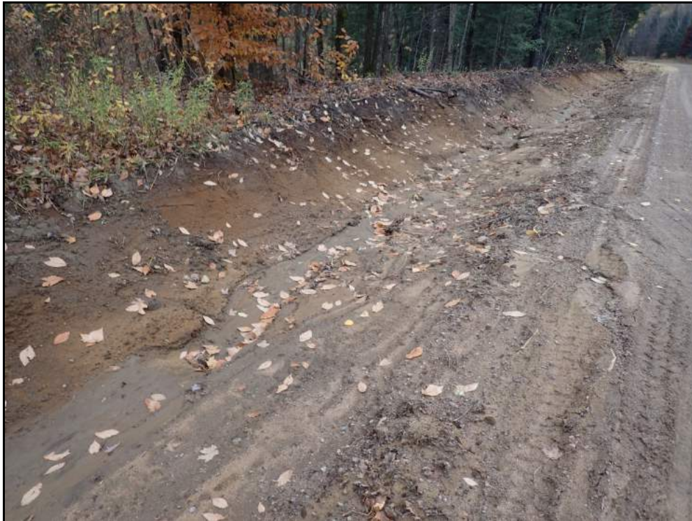
Figure 3.12: Recently excavated roadside ditch along Maple Road. Fine sands are easily transported down-slope.
