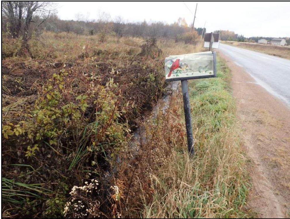
Figure 3.9: Undercut road embankment. Alderdale Road at River Road – Graham Creek.
