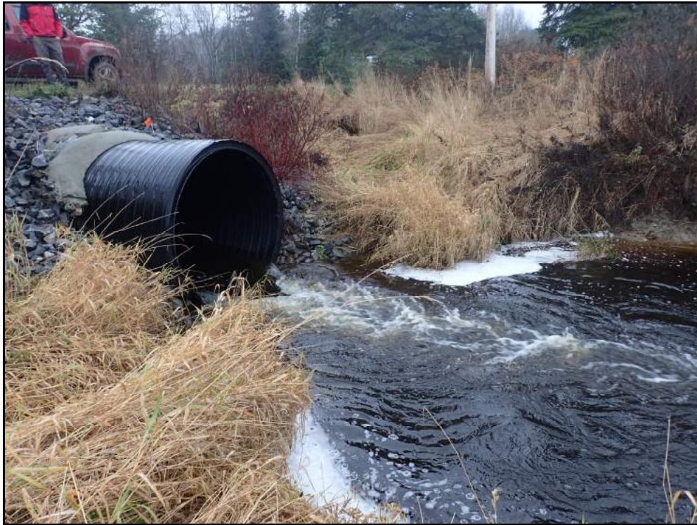
Figure 3.3: Pinecreek Road culvert outlet. Note the perched culvert.
