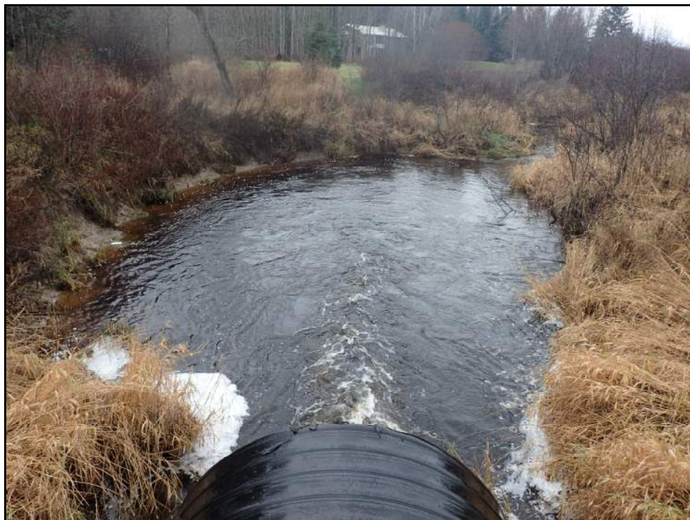
Figure 3.2: View downstream from Pinecreek Road and eroding left bank.
