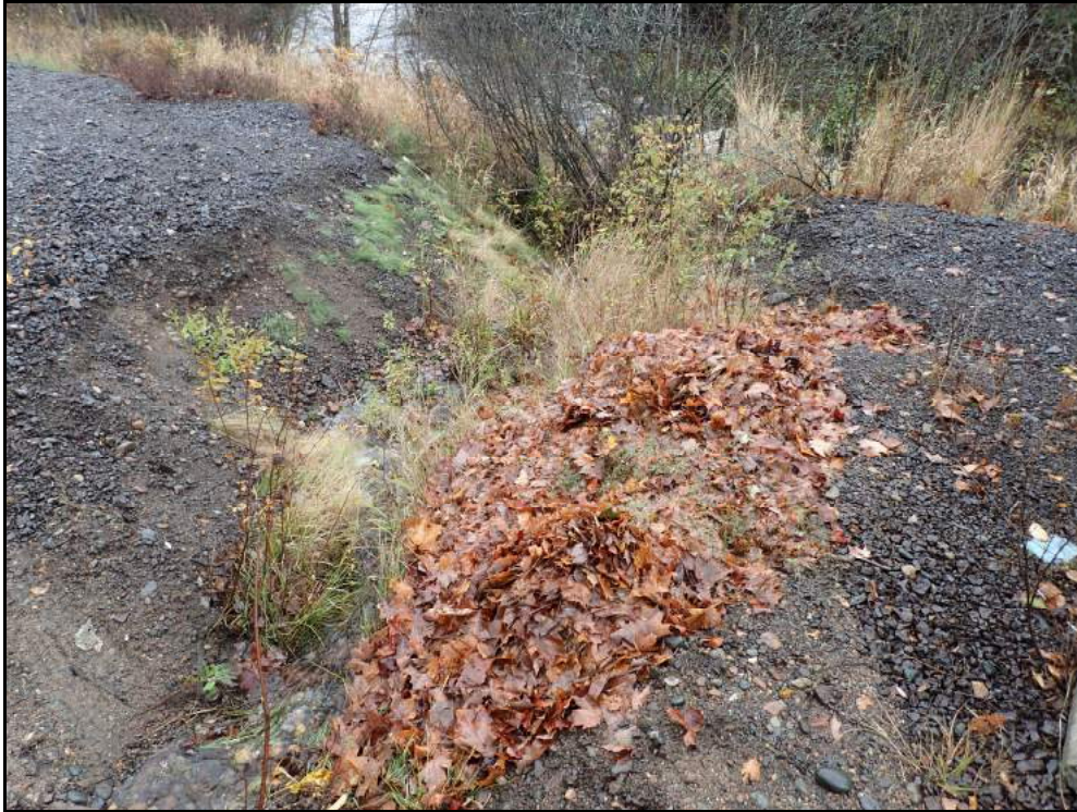
Figure 3.4: Gullying into rail embankment (photo taken leaning over barrier).
